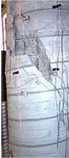
Photo: 1 Failed Column
